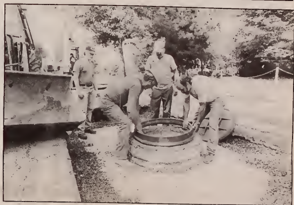
Under construction... Workers from Stone Valley Construction Co. finish raising the manholes on Pollock Road at University Park as part of the construction project for installation of telecommunication lines and electrical duct banks that will provide service to the expansion of West Campus. The construction is expected to be completed next month.
